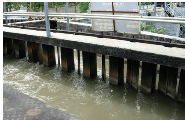
Fig. 18.4 Grit and sand removal tank
