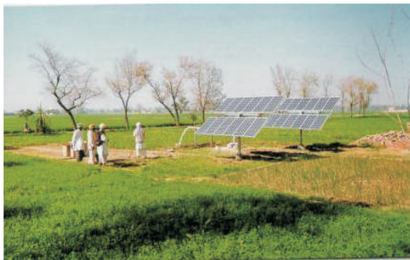
Fig. 12.2 Photovoltaic Water Pumping
