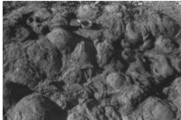
Fig.6.4 : Exfoliation (Flaking) and granular disintegration
